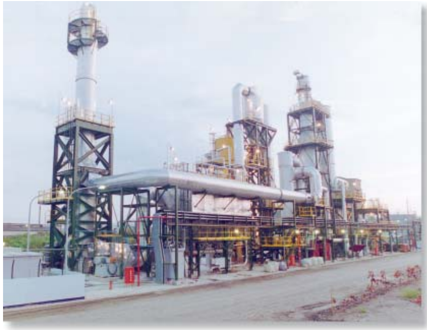
AirPol Air Pollution Control System for a hazardous waste incineration plant in Taiwan.
