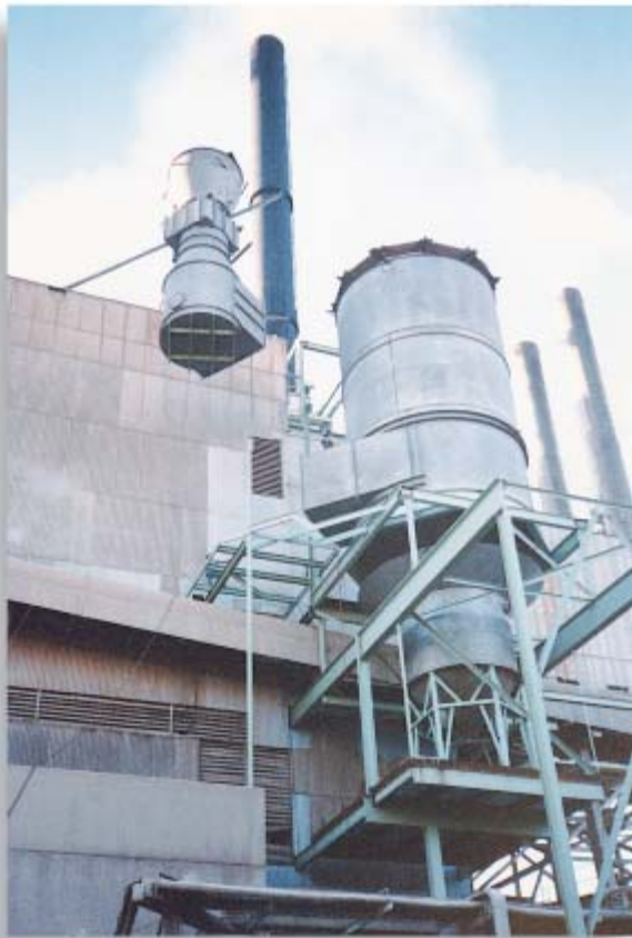
Installation of "Turnkey" AirPol Power Boiler Venturi Scrubber System to handle 275,000 ACFM.
