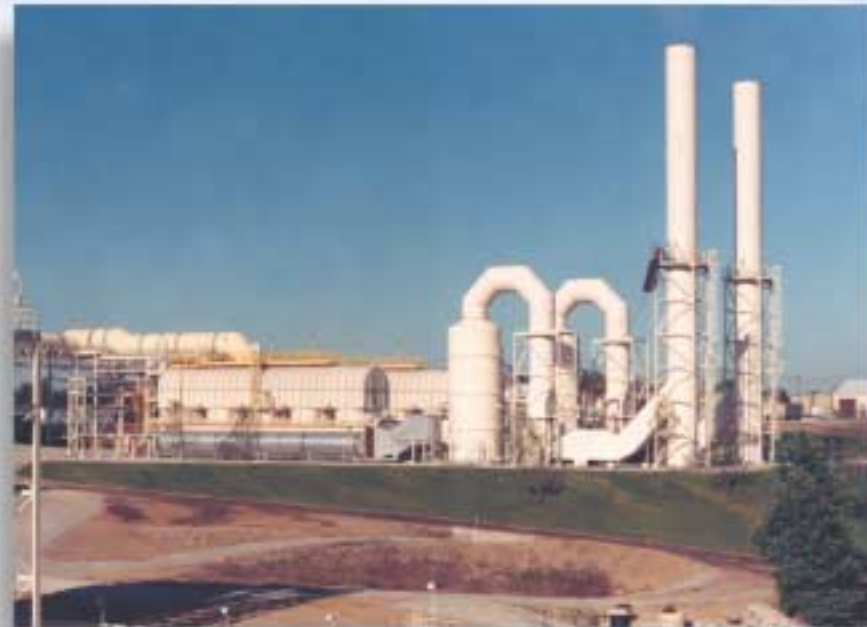
Two FRP Absorption Systems for a Hazardous Waste Thermal Oxidizer
